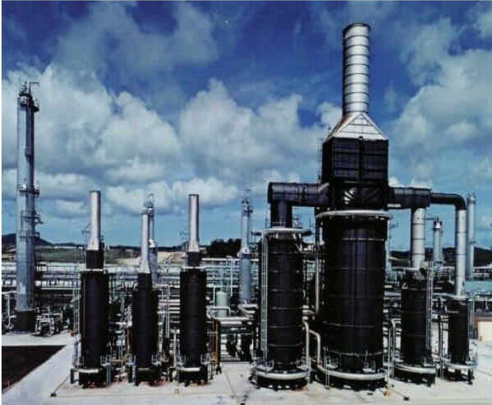
378 M 3 33,000 BPD Reformer Heaters
