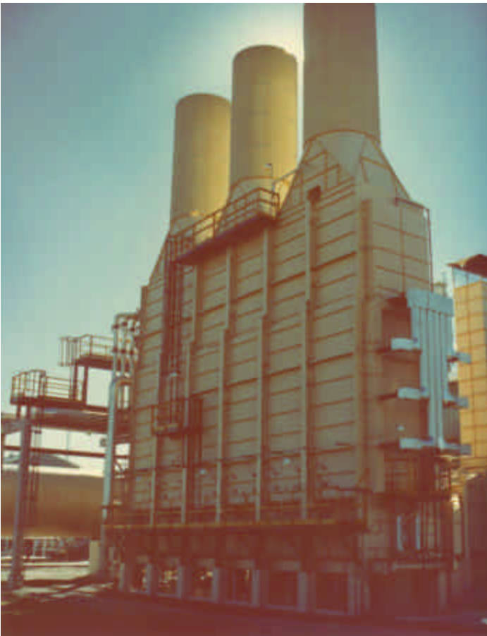
125,400,000 BTU/Hr Radiant / Convection Process Furnace
